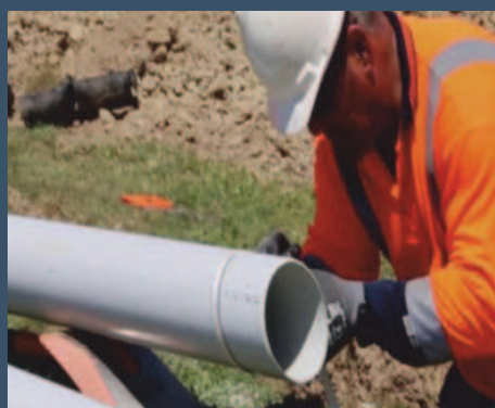
Underground Water Supply Pipeline
