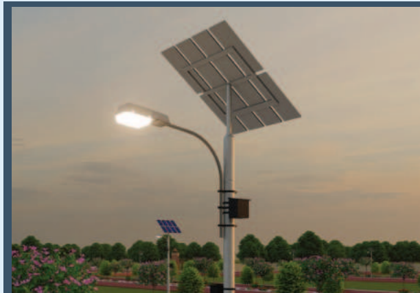
Solar Street Lights
