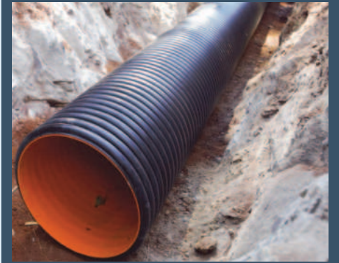
Underground Sewer Pipeline
